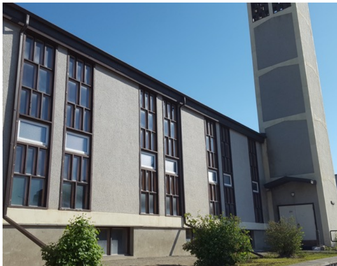
Figure 3: View of windows on south side of building. Note the newer white awning windows within the original coloured glass cathedral window assemblies. Photo supplied by Northern Climate Engineering.
