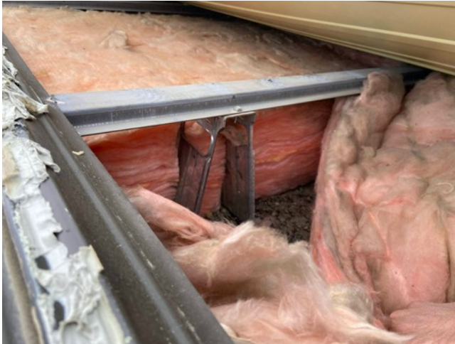
Figure 2: View of retrofit fiberglass insulation on the roof. Photo provided by Doug MacLean.
